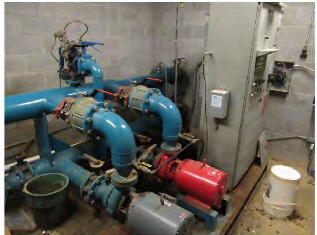
Irrigation pumps and controls overview – Note: Stonehaven Course
