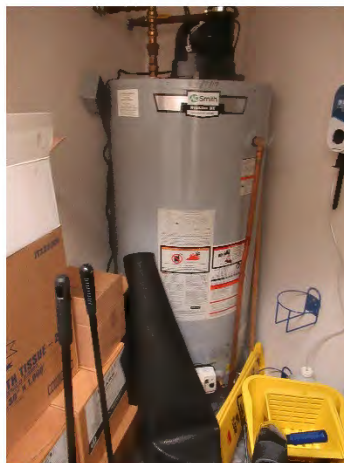
Water heater overview
