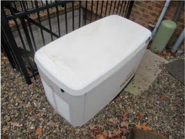
Emergency generator overview
