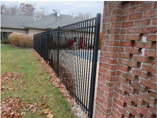
Aluminum fence overview
