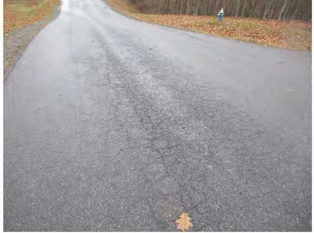
Asphalt pavement cracks
