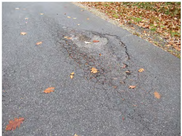
Asphalt pavement cracks and deterioration
