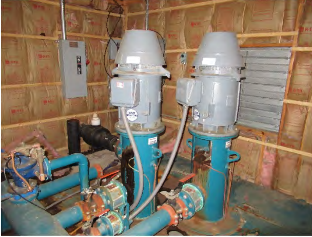
Irrigation system pumps overview – Note: Woodhaven Course
