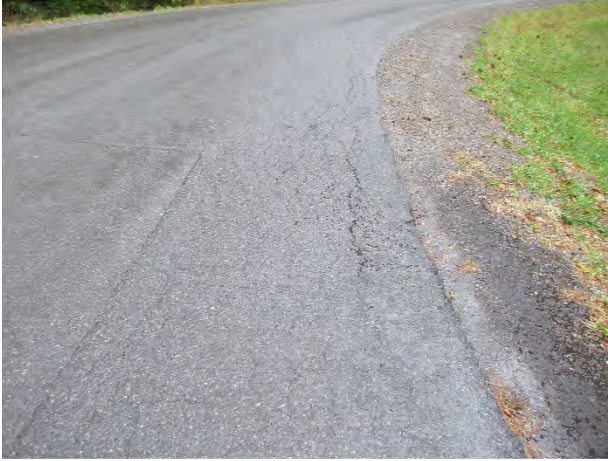
Asphalt pavement cracks
