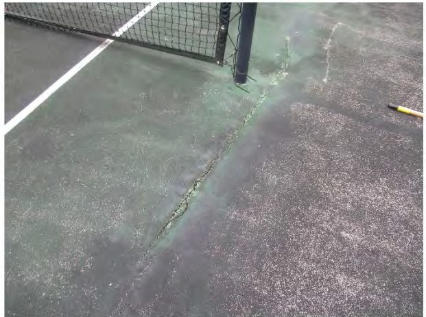
Surface wear and deterioration
