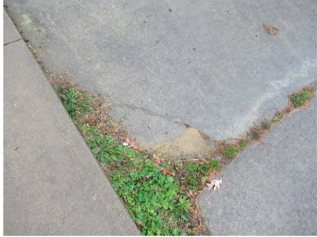
Concrete boat launch crack
