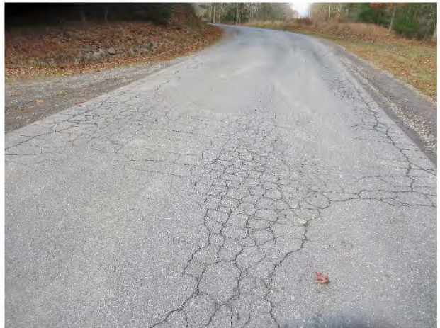
Asphalt pavement cracks and deterioration
