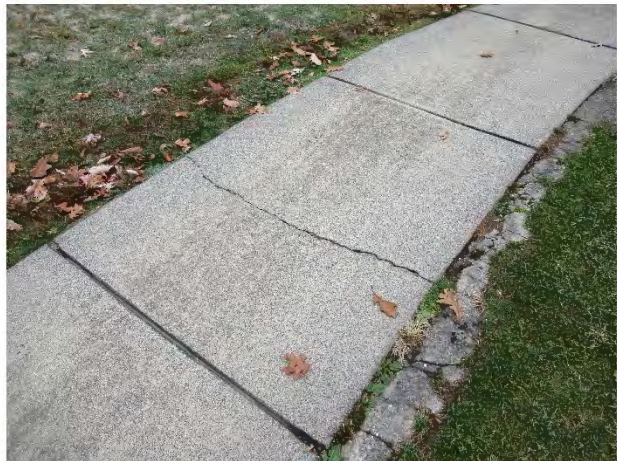
Concrete cart path crack – Note: Woodhaven Course
