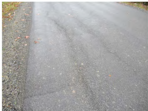
Asphalt pavement cracks
