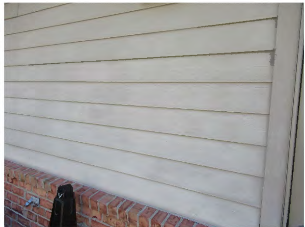
Fiber cement siding finish deterioration
