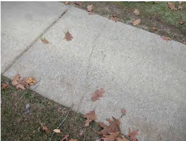
Concrete cart path crack – Note: Woodhaven Course
