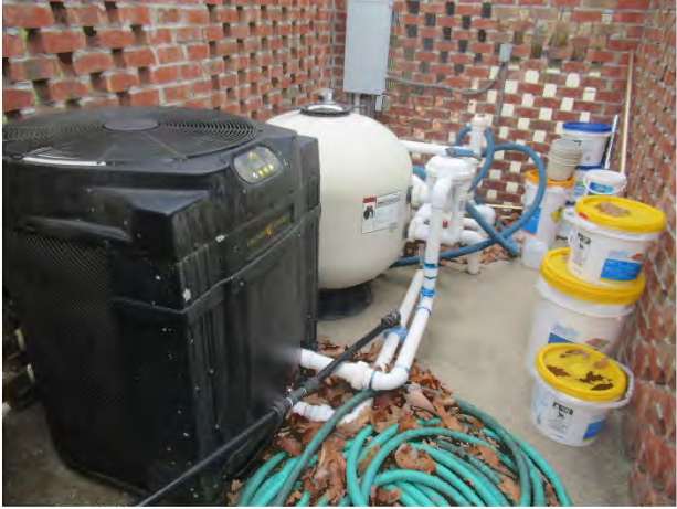
Pool mechanical equipment overview
