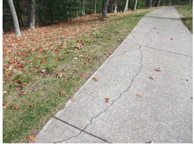
Concrete cart patch cracks – Note: Stonehaven Course
