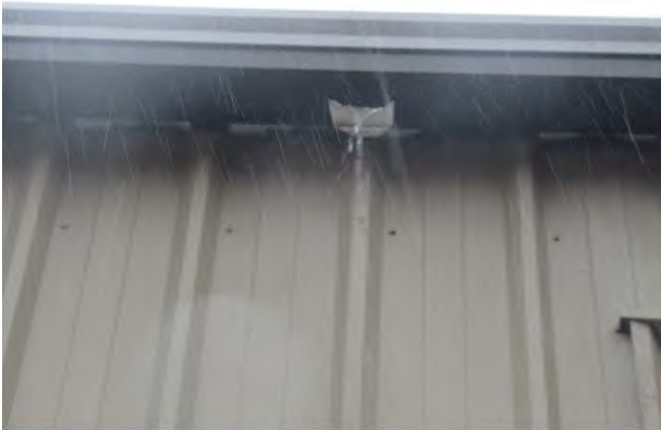
Missing downspout – Note: Stonehaven maintenance building
