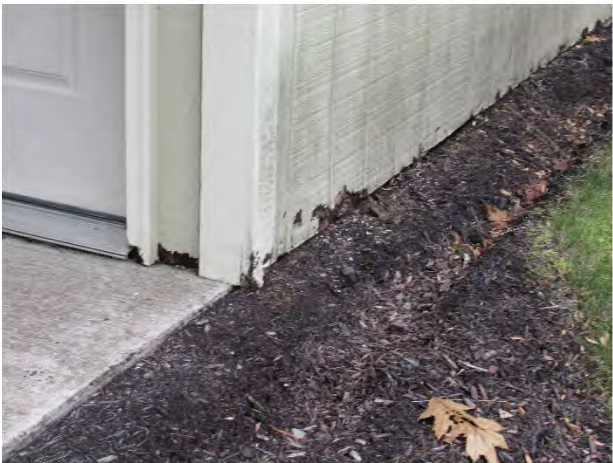
Siding damage and stains – Note: Woodhaven Course
