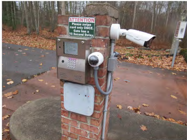
Rear entrance gate entry system
