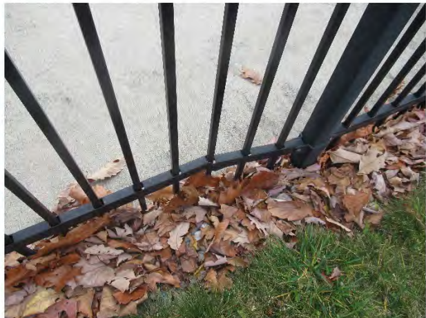
Aluminum fence damage
