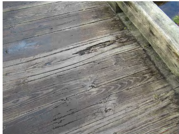
Wood cart path bridge deterioration – Note: Stonehaven Course
