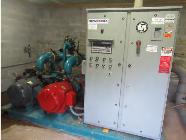
Irrigation system pumps and controls
