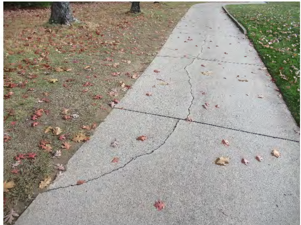
Concrete cart patch cracks – Note: Stonehaven Course
