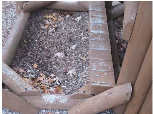
Playground equipment wear
