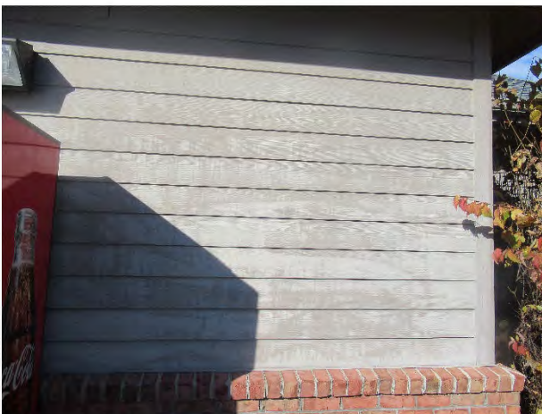
Fiber cement siding finish deterioration
