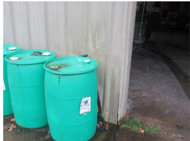
Metal siding damage – Note: Stonehaven maintenance building
