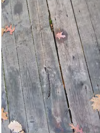
Wood cart path bridge deterioration – Note: Stonehaven Course
