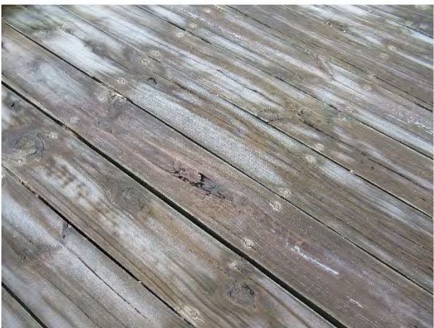
Wood cart path bridge deterioration – Note: Woodhaven Course
