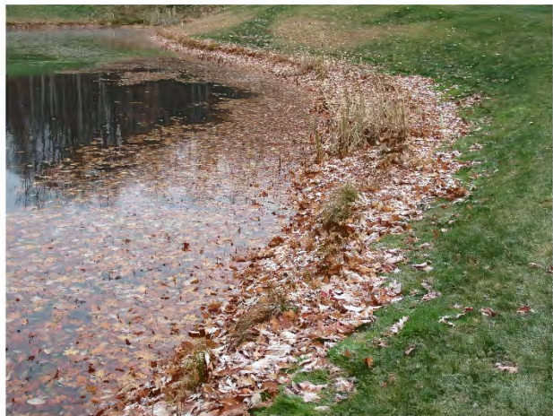
Sediment accumulation at hole #4 pond – Note: Woodhaven Course
