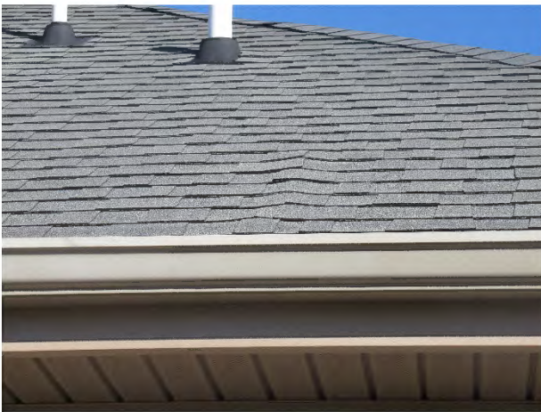
Isolated shingle lift
