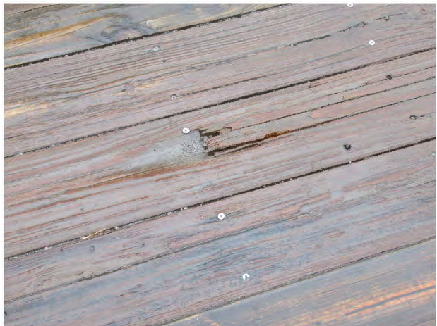
Deck board deterioration
