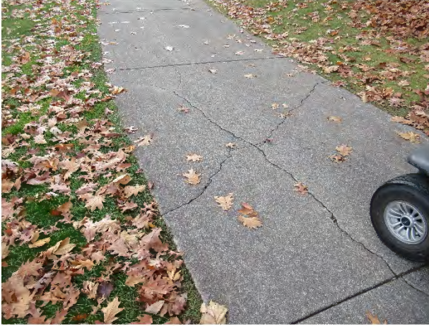
Concrete cart patch cracks – Note: Stonehaven Course
