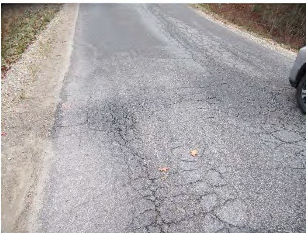
Asphalt pavement cracks and deterioration
