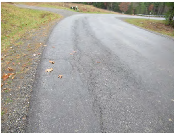
Asphalt pavement cracks
