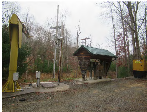
Lift station overview
