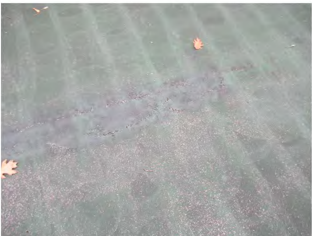
Surface wear and deterioration
