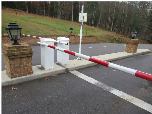
Gates and gate operators at security gate
