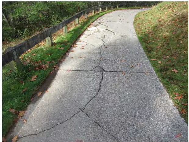
Concrete cart patch cracks – Note: Stonehaven Course
