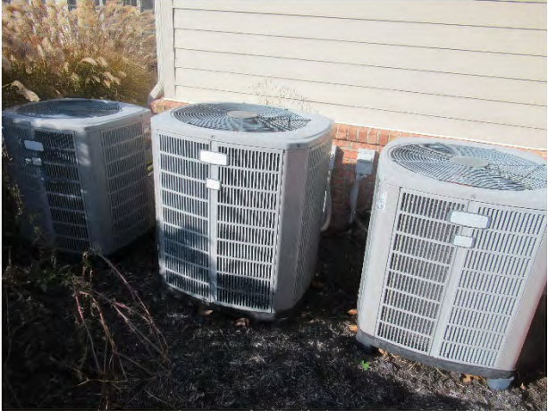
Condensing units overview
