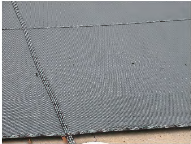
Pool cover damage
