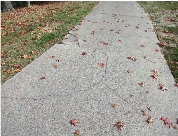
Concrete cart patch cracks – Note: Stonehaven Course
