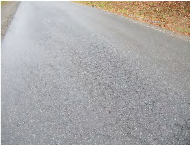
Asphalt pavement cracks
