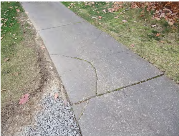
Concrete cart path cracks – Note: Woodhaven Course
