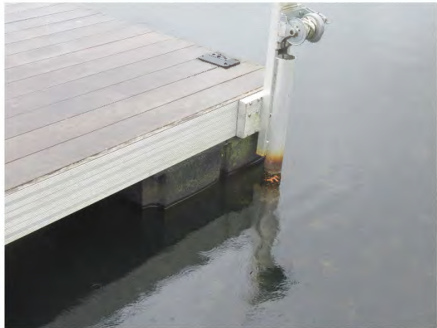
Minor rust at floating dock
