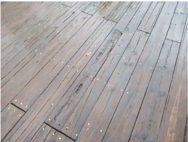
Deck board deterioration
