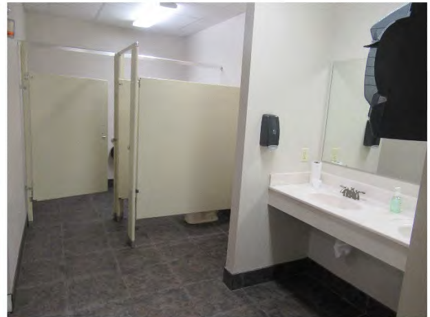
Locker room fixtures
