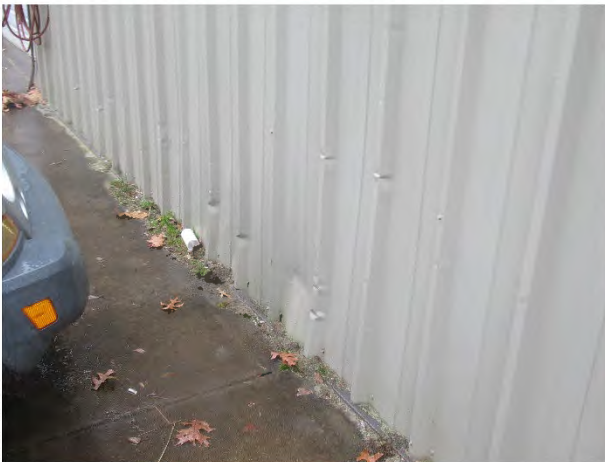
Metal siding damage – Note: Stonehaven maintenance building
