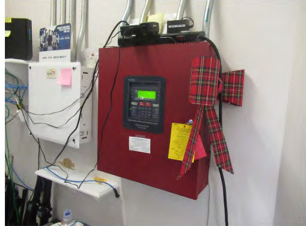
Life safety system control panel
