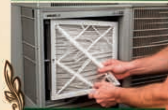
HVAC FILTER CHANGE
