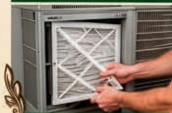
HVAC FILTER CHANGE
